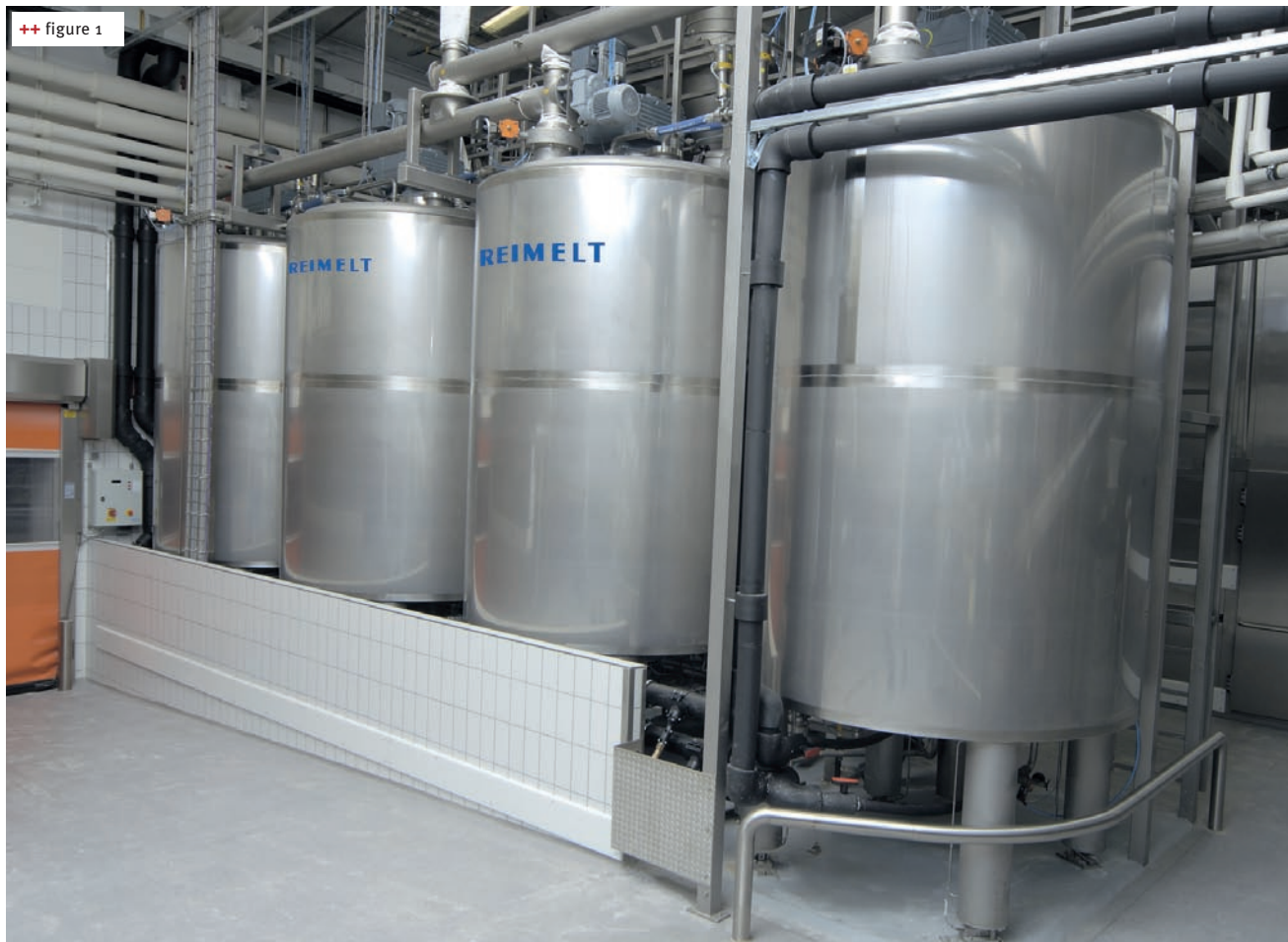
++ figure 1 Silos for liquid components
