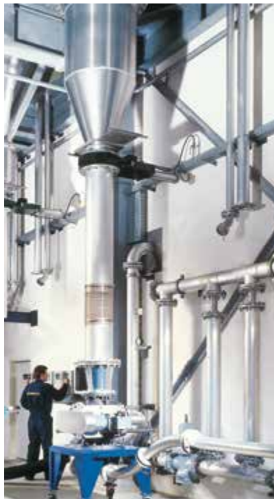
Conveying of pellets by a rotary feeder installed below a blending silo.
